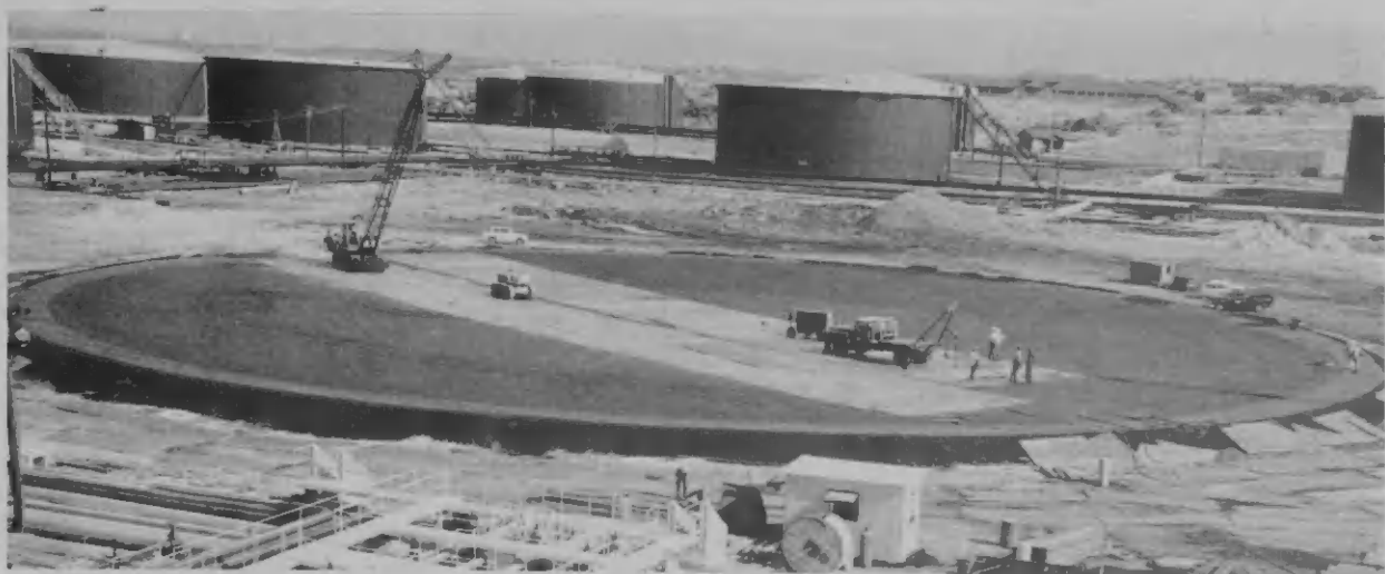
THIS FOUNDATION of a huge crude tank with other tanks in background may give an idea of its size.
